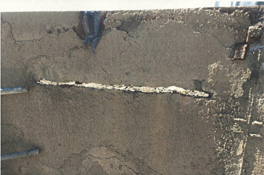
Figure 8 - Internal Picture of Hole in Tank Wall Due to Weather Exposure
