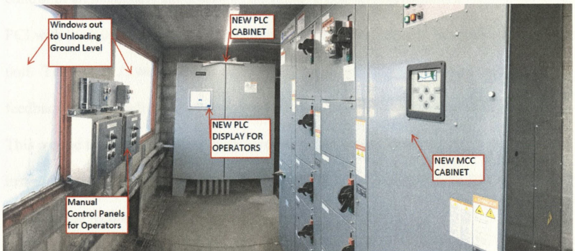
Figure 18 - New Unloading Building Control Room
