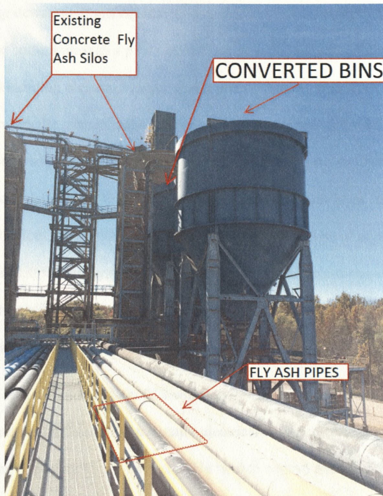
Figure 4 - Photo Looking South at Converted Dewatering Bins
