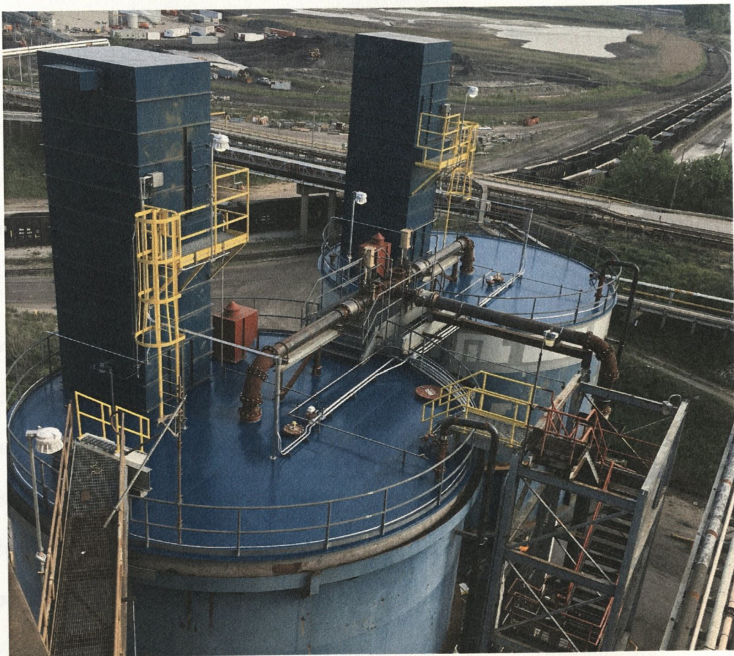
Figure 15 - Rooftop Photo of the Newly Converted Bins with Installed Rooftop Equipment
